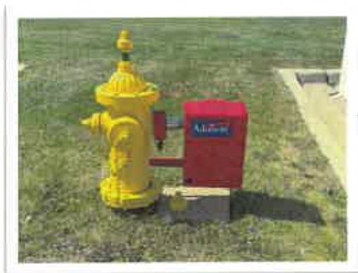
Automatic Hydrant Flusher
